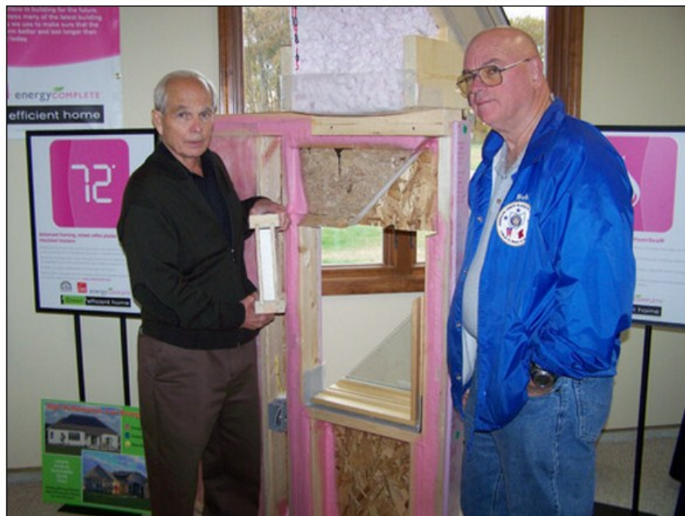
Bill Decker of Decker Homes, left, shows the insulated header concept to Bob Schmitt in a model home at Deer Valley.
